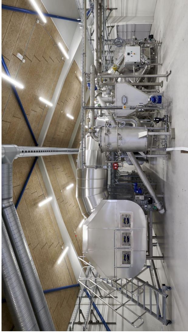
HECLA® Setores 1.000 at Fårevejle Wastewater Treatment Plant
